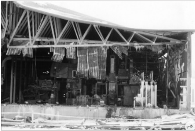
Figure 1 - Destruction from a Dust Explosion in a Paper Shredding Operation. An arrow points to the ruptured dust collector.
